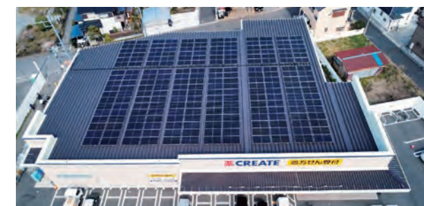
Solar panels installed on store rooftop
